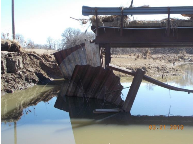
Damage: Loss of abutment wall. Solution: construct new abutment wall. Will likely require stiffer sheeting and a dead man. Status: Preliminary, going to site visit today to do further evaluation with water down. Will develop repair plan and obtain quotes. Cost estimate: $130,000
