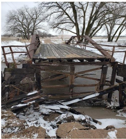
Damage: Loss of abutment wall and fill. Solution: construct new abutment wall. Will likely require stiffer sheeting and a dead man. Status: Will develop repair plan and obtain quotes. Cost estimate: $130,000
