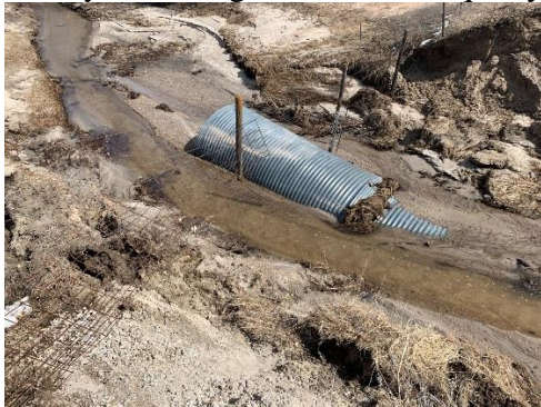
Damage: Loss of roadway approach and culvert pipe. Solution: replace with new bridge. Pipe too small for crossing. Status: Waiting to meet with FEMA and Knox County to discuss options. Cost estimate: $500,000; County share would be split with Knox County
